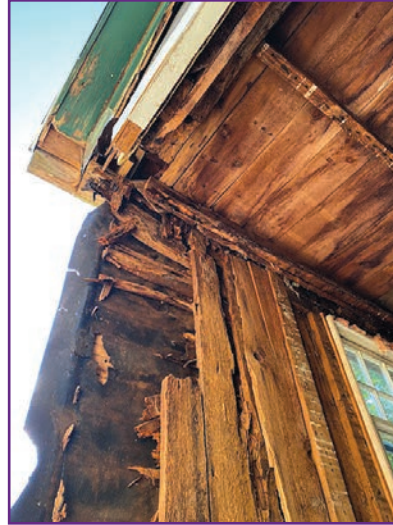
Interior damage Photo: Jim McIntire
