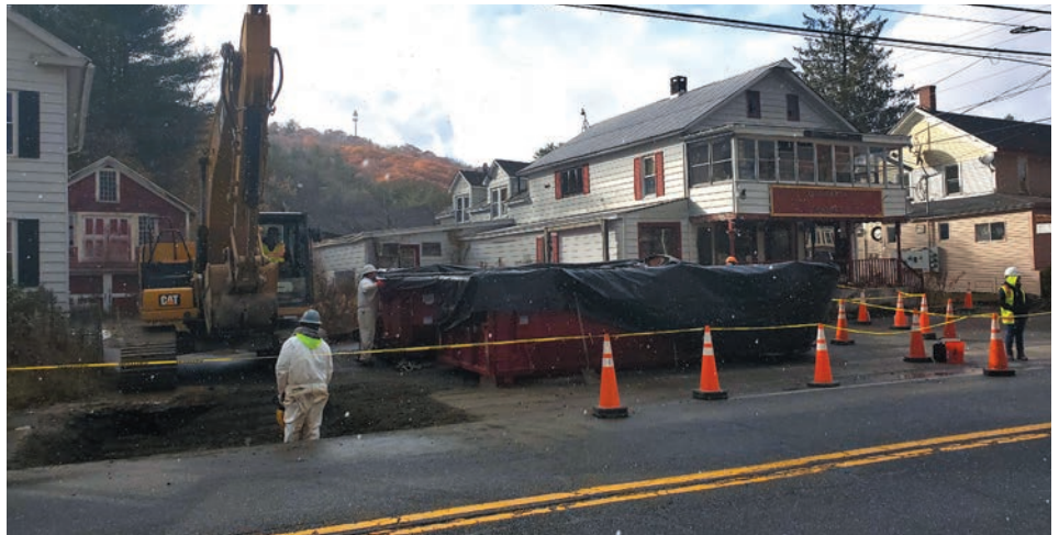
The Massachusetts Department of Transportation (DOT) is pictured here installing catch basins in front of the abandoned Terranova property on Route 8, just south of the town center. Recent sidewalk upgrading (also done by the DOT) altered the pitch of the roadway which often led to flooding on Main Street. The catch basins will capture and redirect any excess water away from the roadway.
